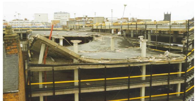
Figure 4. Punching Shear Failure [12]
