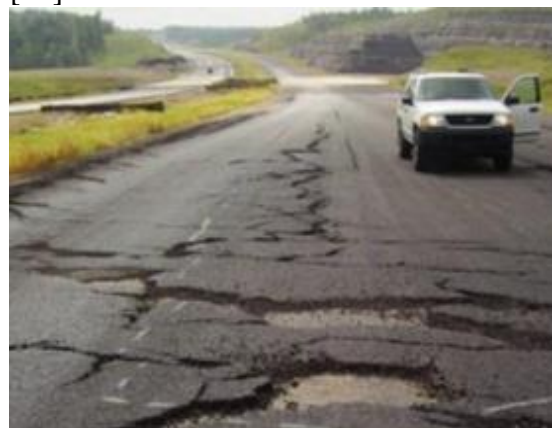
Figure 1. Delamination interface failure [22]
